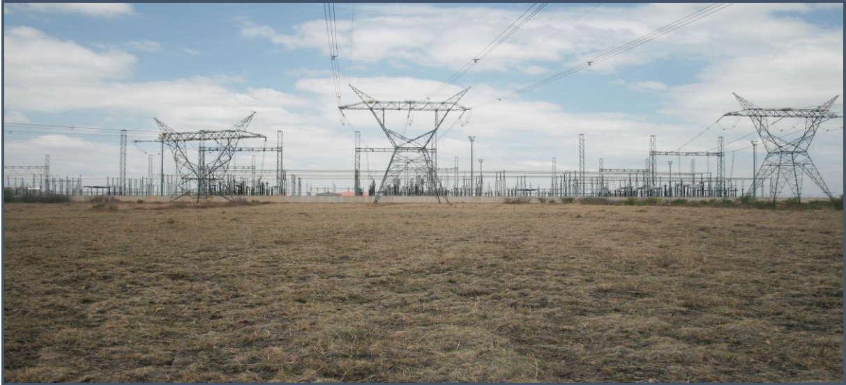
Figure 3: Bighorn –Marang and Medupi-Marang 400kV power lines feeding into Marang MTS
